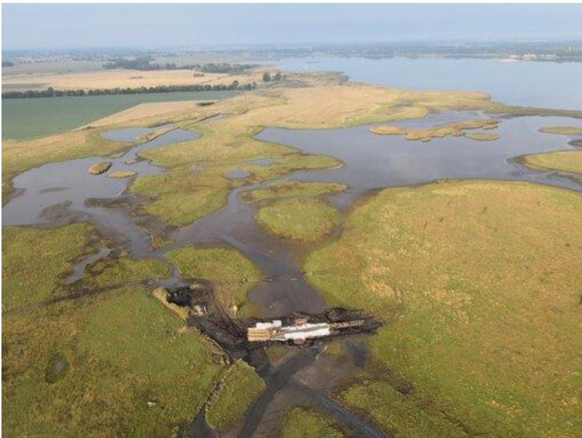
Fig. 5. Construction measures to revitalise natural processes in the Karrenderfer Wiesen near Greifswald, seen from a crane’s perspective (Photo: N. Seifert / Michael Succow Foundation).
